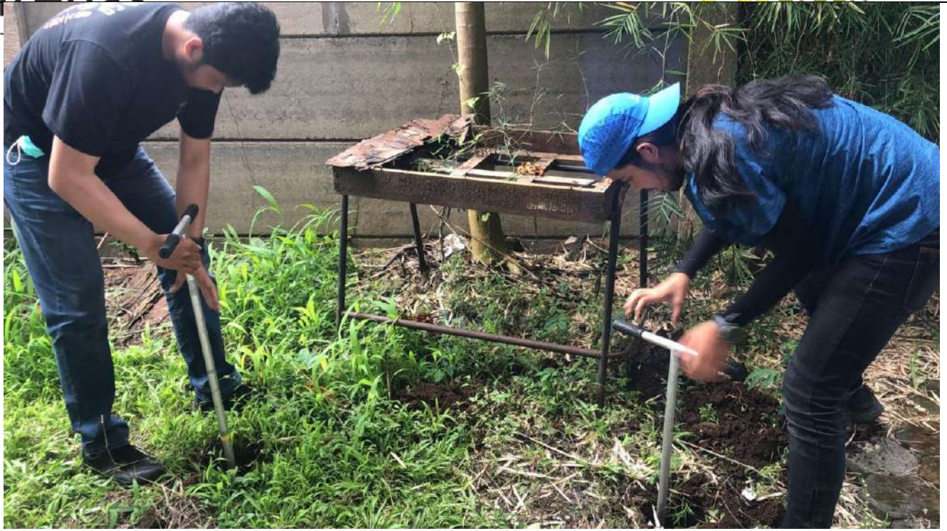
Building SWG in Bandung areas
